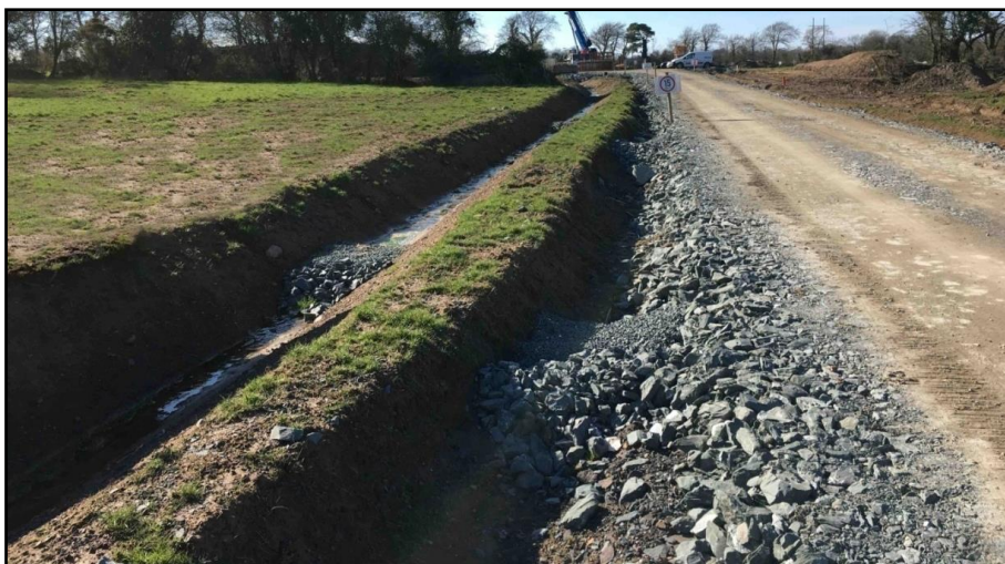
Plate 2-1: Example of conveyance swales and vegetated soil bund
