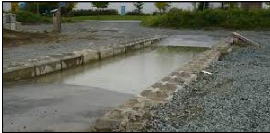
Plate 3-13: Example of the multiple variations of wheel wash used on wind farms
